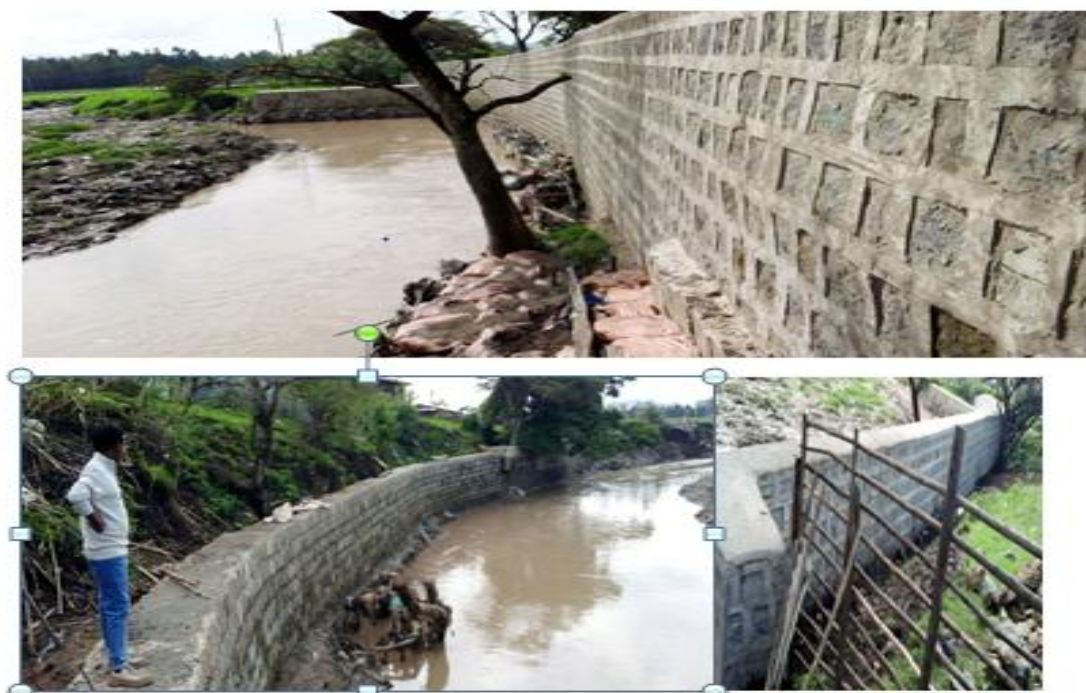
Figure 10 Flood Walls Found in Akaka Sub City.
