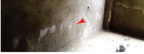
Fig. 4.11 Efflorescence in interior wall in sample site
