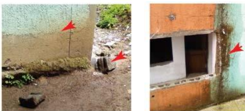
Fig. 4.10 Discoloration, Plaster debonding and fungus effect on masonry work
