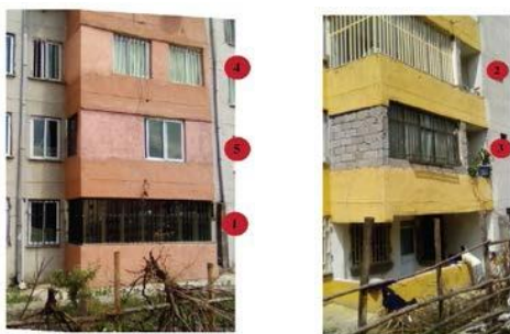
Fig 4.6 Balcony engulfed to the interior
