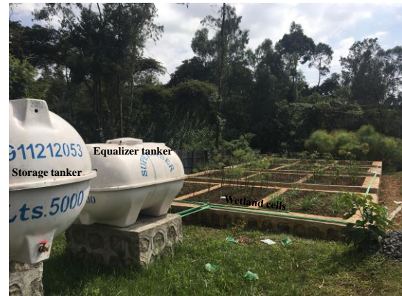
Figure 1: Wastewater treatment system (field view) at NALRC
