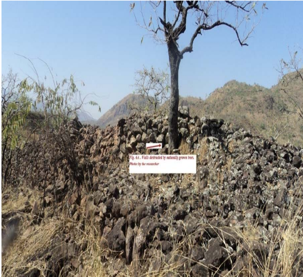
Figure 6: The wall structure cracked by naturally grown trees (photo by the researcher)
